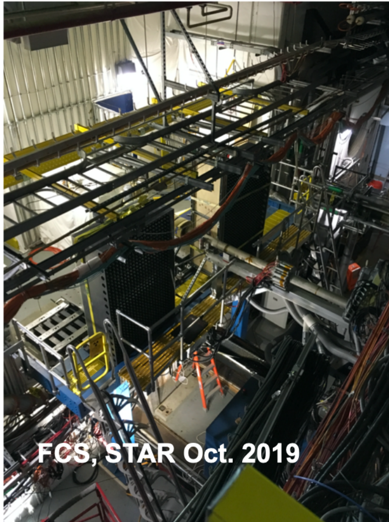
Figure 91: A view of the installed forward ECal detector halves, left and right from the beam pipe.
